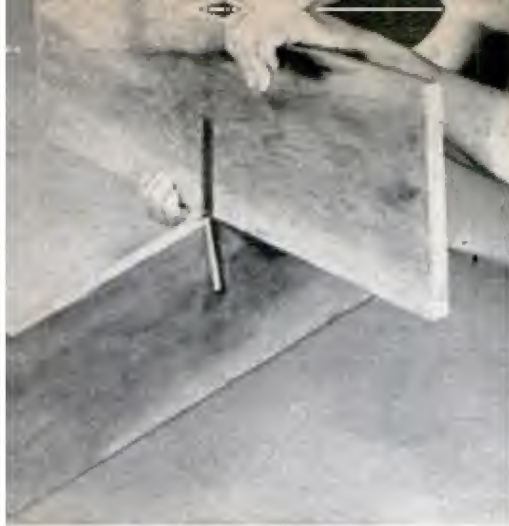
CROSS BRACES are joined, using a snug half-lap joint. Apply glue generously to the mating surfaces
